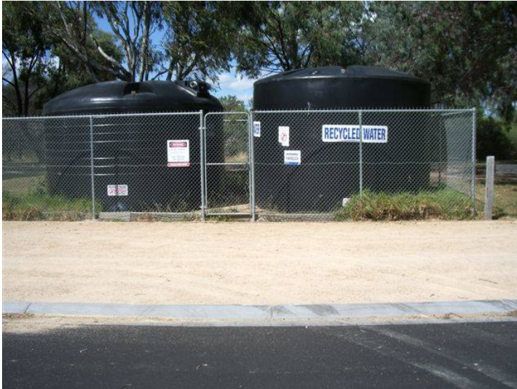
Minor Storage tanks
