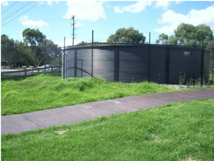
Major 230KL tank to store harvested water for irrigation
