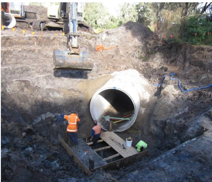
2.4m diameter storage pipes for stormwater harvesting
