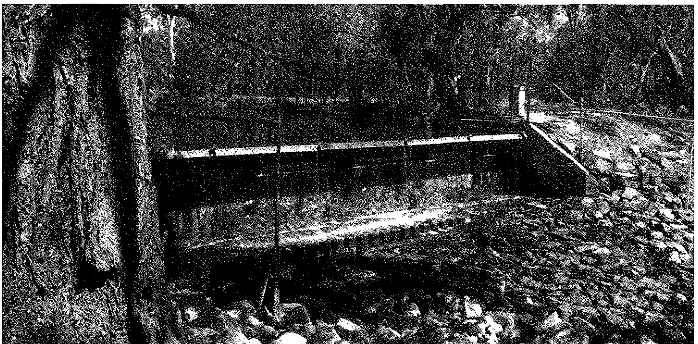
Water flows over the newly refurbished Quambatook Weir for the first time. PHOTO: GANNAWARRA SHIRE COUNCIL
